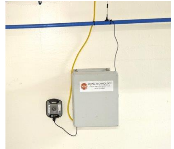
Vibration monitor installed in basement
