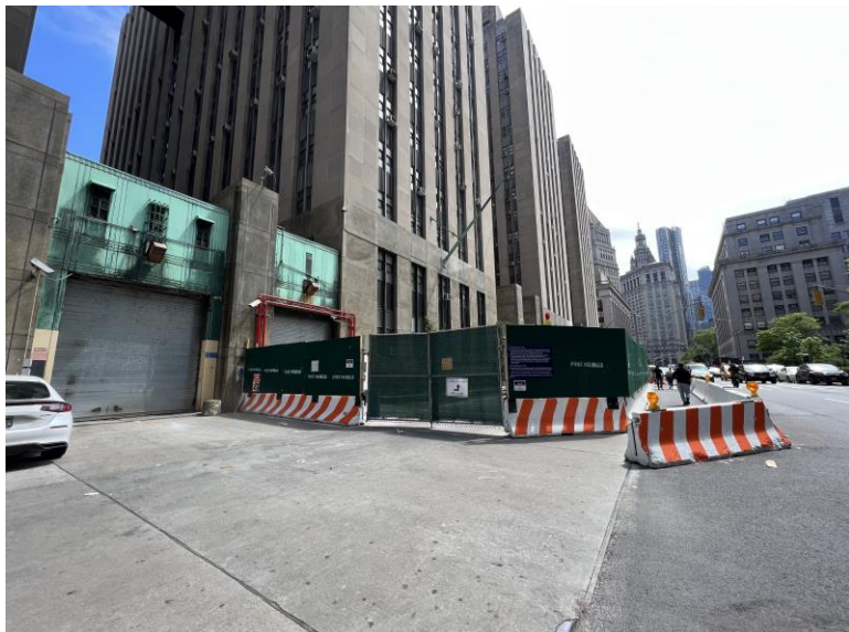
Site Protection Fence to the New Interim Sally Port (6/14/2022) 臨時安全通道保護圍欄 (6/14/2022)
