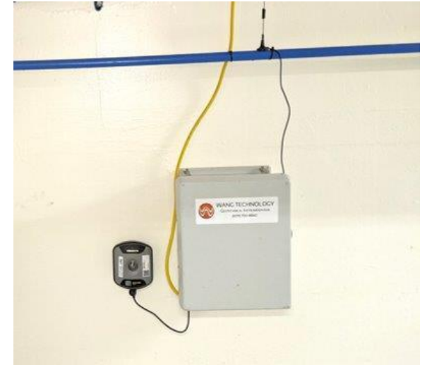
Vibration monitor installed in basement
