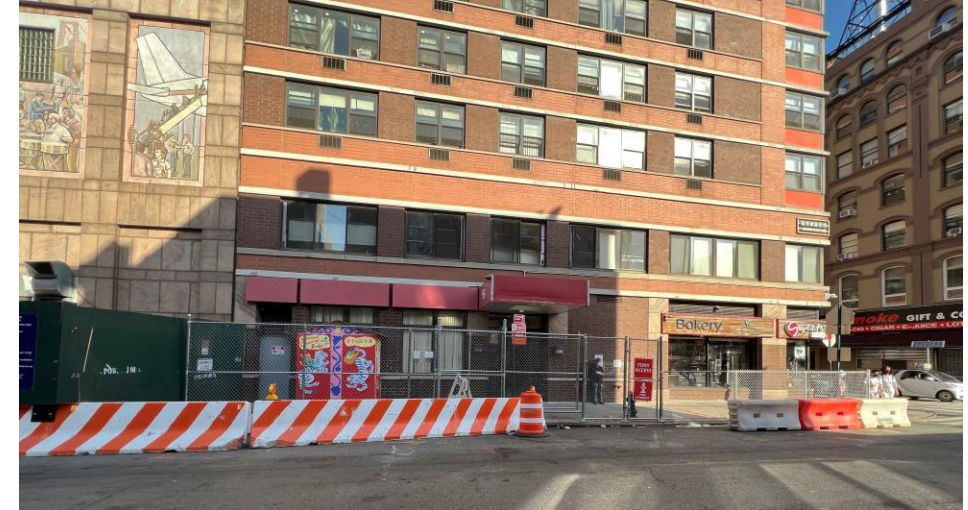
Construction Fencing on Baxter Street (7/21/2022) Baxter Street/巴士特街施工保護圍欄(7/21/2022)
