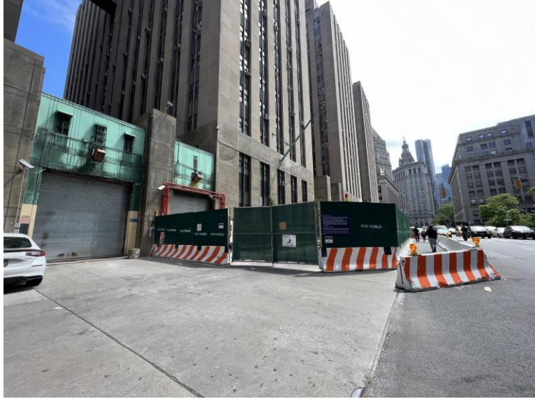
Site Protection Fence to the New Interim Sally Port (7/21/2022) 臨時安全通道保護圍欄(7/21/2022)
