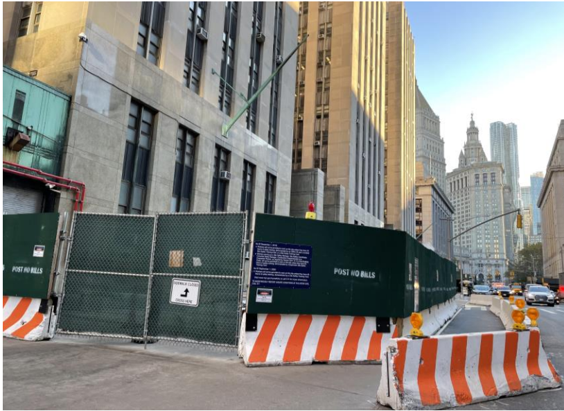
Site Protection Fence to the New Interim Sally Port (11/21/2022) 臨時安全通道保護圍欄 (11/21/2022)
