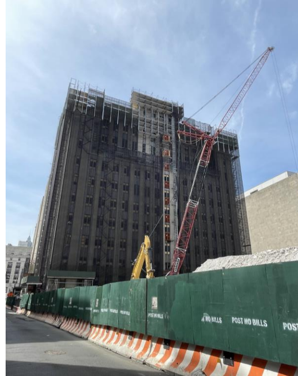
North Tower Dismantlement and South Tower Scaffolding Installation 北樓拆除現況和南樓安裝鷹架 (4/9/2024)
