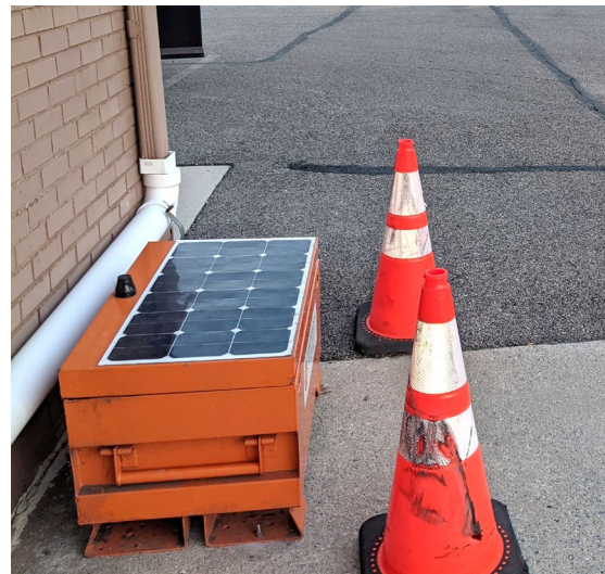
Vibration monitoring installed outside on sidewalk
