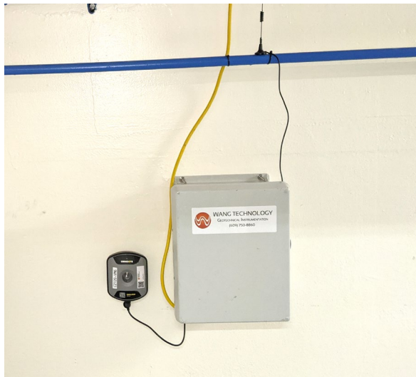
Vibration monitoring installed in basement
