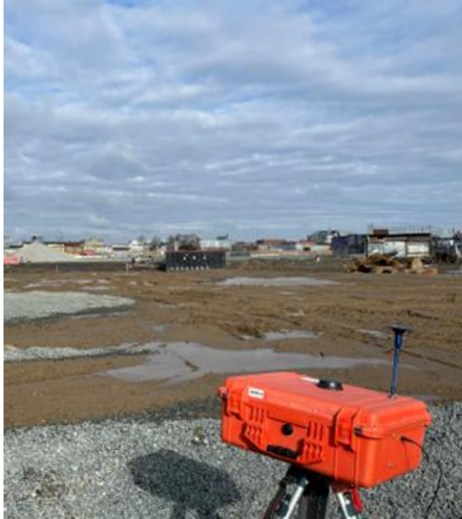
Air Monitoring Station
