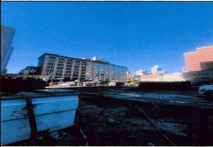
Photo 7: View of site looking northwest showing damp/wet ground due to misting/water suppression activities, 11/13/24
