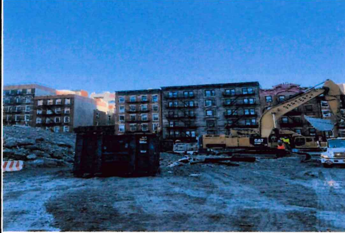
Photo 9: View of site looking east showing damp/wet ground due to misting/water suppression activities, 11/13/24
